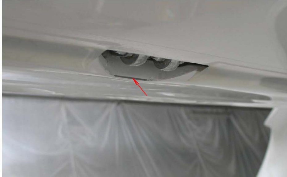
Fig. A: Inspection area: Trim tab control horn attachment point (Seen from underneath the stabilator)
